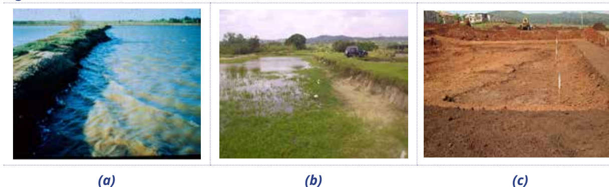
Figure 17: Erosion of Pond Walls
